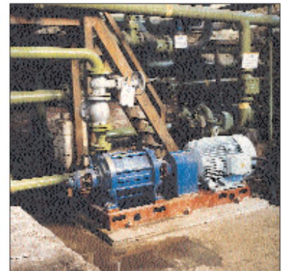
This five stage multi-stage pump is used for pumping water to a hill top reservoir for British Steel
