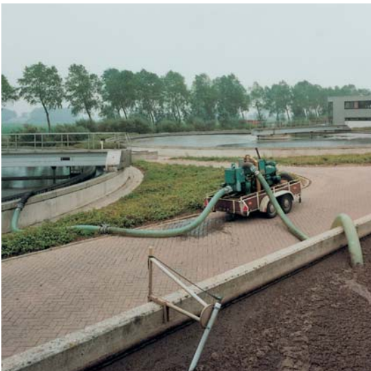
Emergency pump (VRP) for sewage treatment plant.
