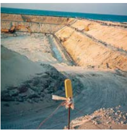
Dewatering of deep and large construction sites in the Netherlands and abroad.
