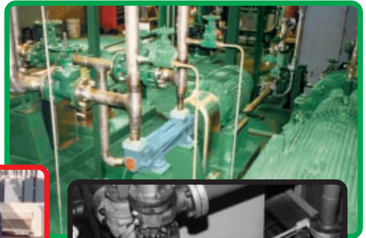
12D-137 pump on compressor gas sealing service
