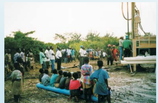
Drill rigs will be needed for areas that cannot install the SolarPedalflo on existing wells. In this picture, MWI is demonstrating the process of drilling.
