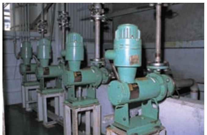
Basic type pumps in a chemical plant.
