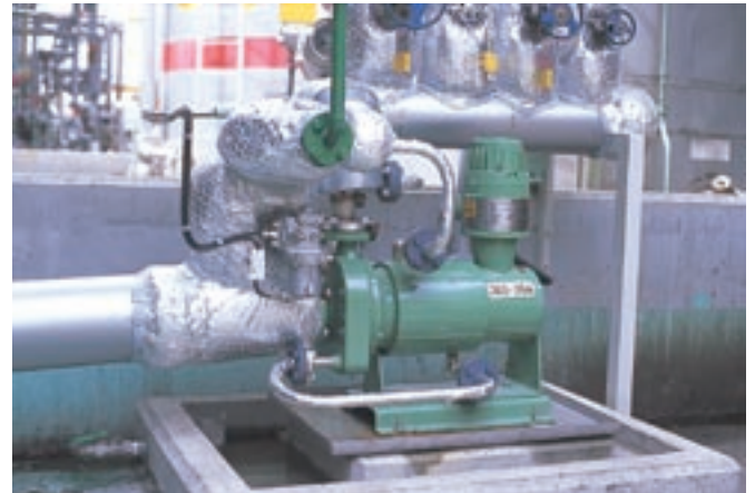
High melting point type pump in a chemical plant.
