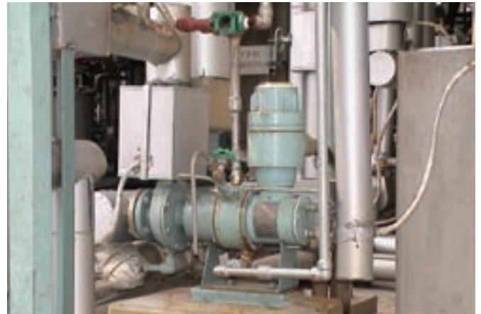
High-temperature type pump in a chemical plant.
