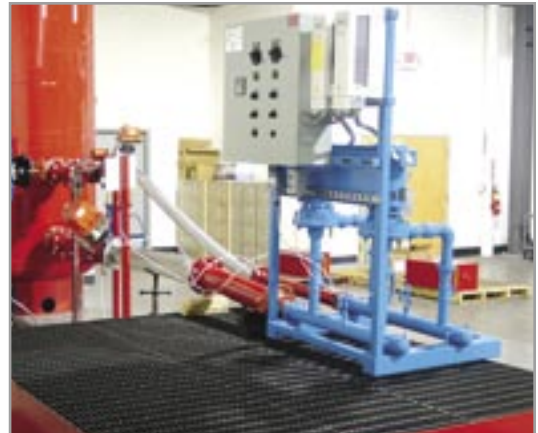
Booster System Undergoing Testing.
