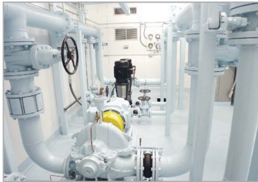
Above Ground Installation.
