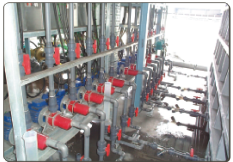
Battery of DC-31 Pumps for dosing application
