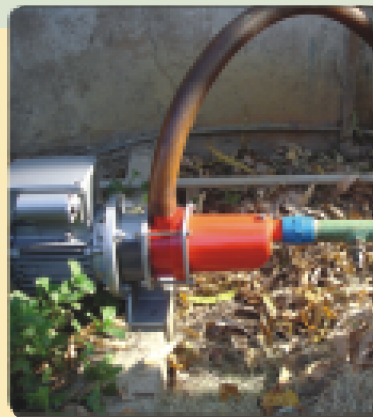
DC-12 Pump for sprinkler system
