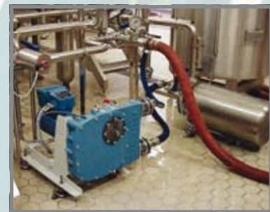
Brewing - Pumping Kieselguhr
