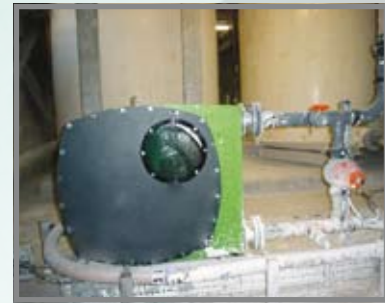
Water treatment - Lime mixing & recirculation
