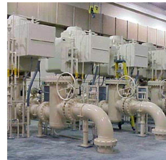
Top: Booster pumps
