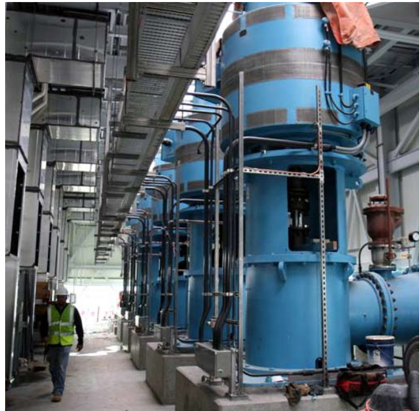
Below: Raw water service pumps
